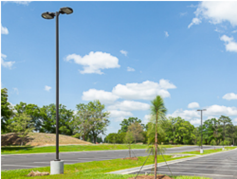
Pole Mounted Double Fixture
