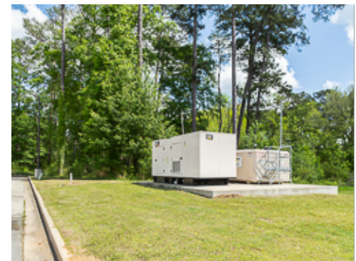
Pad Mounted Equipment
