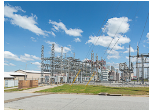
Electrical Substation and Tanks
