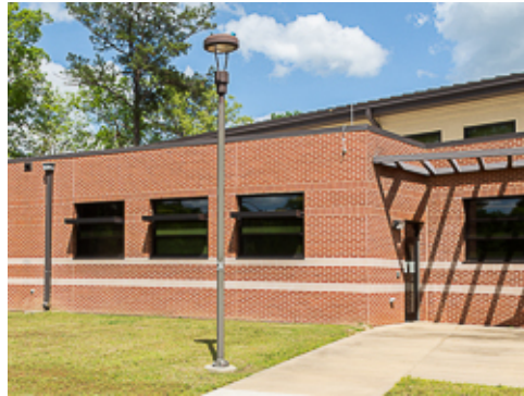
Pole Light at Entry
