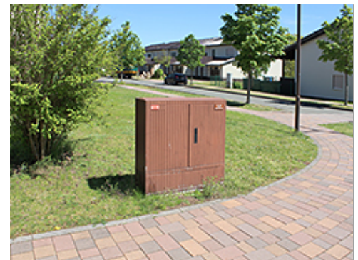
Standard Electrical Cabinet
