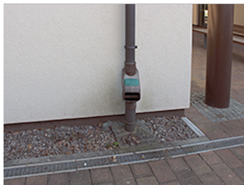
Roof Drainage Connected to Storm Sewer
