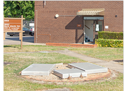
Utility Vault Elements
