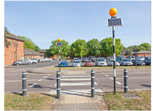
Coordinated Access Control Elements
