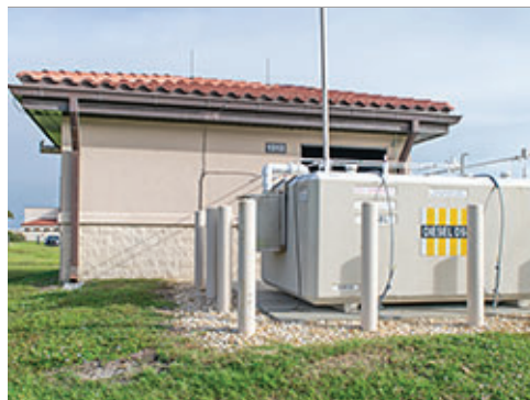
Concrete double walled fuel tank
