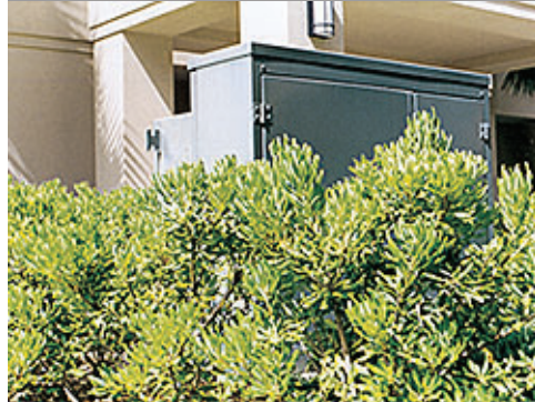
Screened Utility Component
