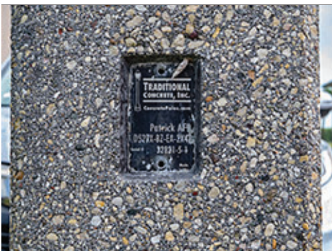
Concrete utility pole
