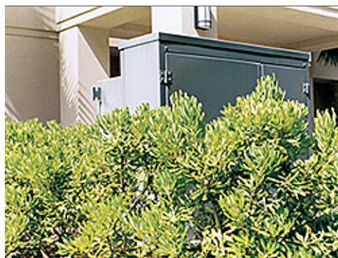
Screened Utility Component
