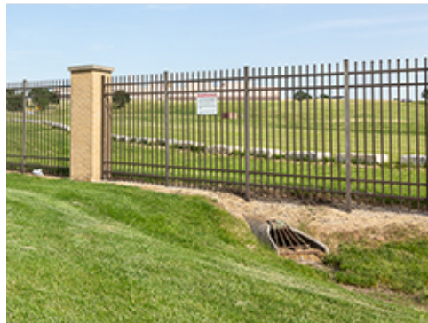
Stormwater Discharge Element
