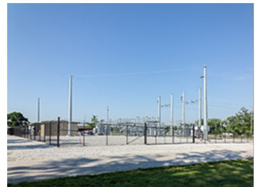
Electrical Service Site in Group 3
