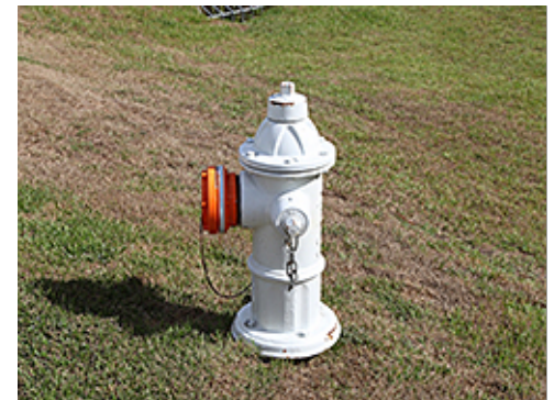
Base Standard Utility Marking
