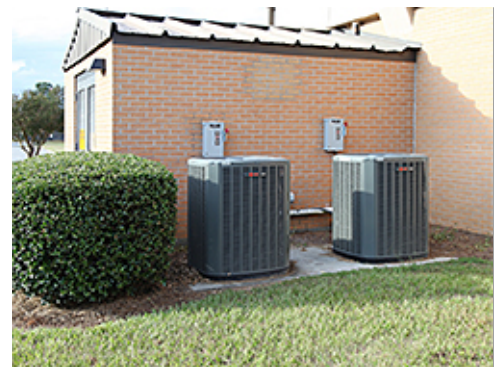
Screening of Mechanical Equipment
