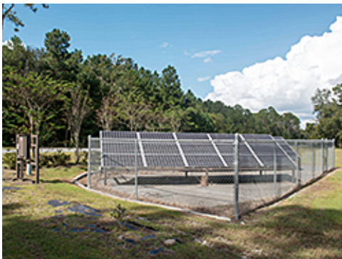
Renewable Energy Solar PV Array
