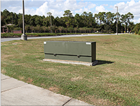
Pad Mounted Cabinet
