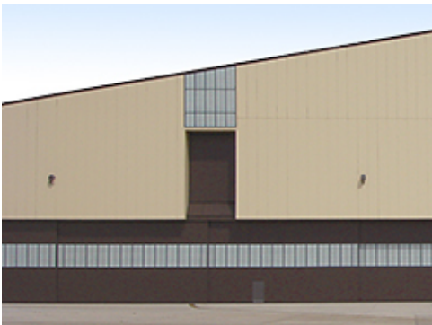
Group 3 Wall Mounted Apron Lighting
