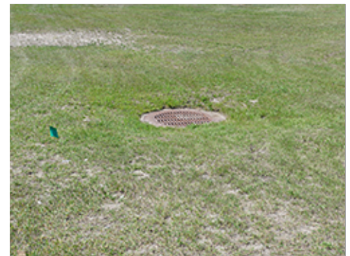
Stormwater Outlet to Detention Area
