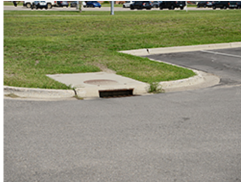
Storm Sewer Inlets with Accessible
