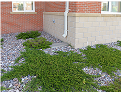
Group 2 Downspout w/Grey Water Irrigation
