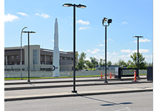
Parking Lot Light Double Mount
