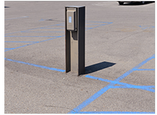
Electrical Access for Vehicle Block Heater
