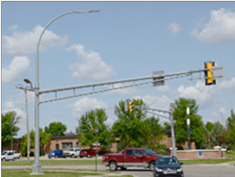
Incorporated Street Lights and Traffic Signal
