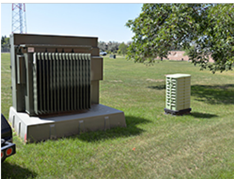
Group 1 - Concrete Pad Mounted Transformer
