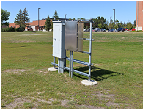
Group 2 - Small Concrete-mounted Utility Box
