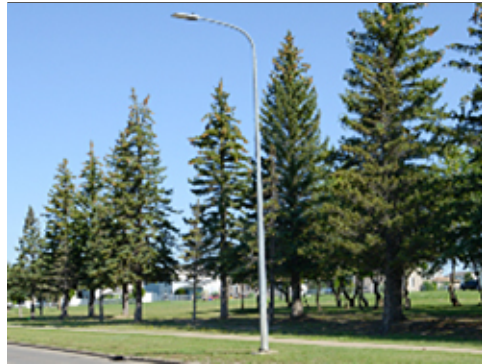
Standard Street Lighting
