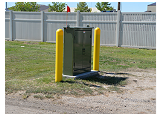
Group 2 Utility Cabinet and Vehicle Bollards
