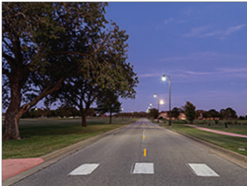
Street Lighting at Crosswalk
