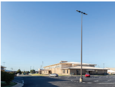
High Mast Lighting
