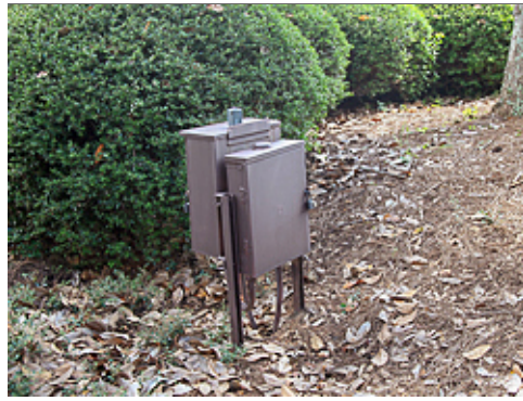
Painted Control Box
