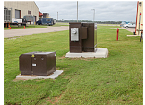
Group 3 Ground Mounted Cabinets
