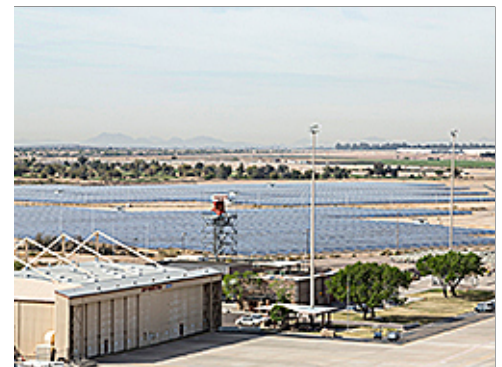
Ground Mounted Solar Array
