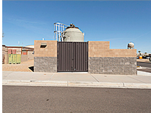
Screen Wall at Utility Equipment
