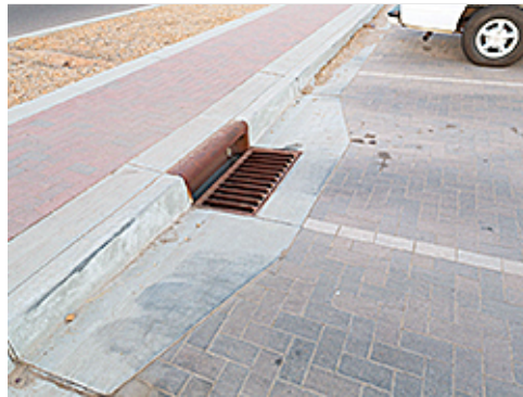
Curb and Gutter Inlet
