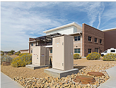
Pad Mounted Electrical Cabinets
