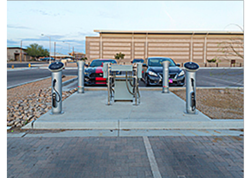
EV Charging Station Gear
