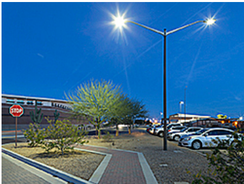
Combined Sidewalk and Automobile Lighting
