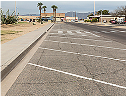
White Striping on Asphaltic Paving
