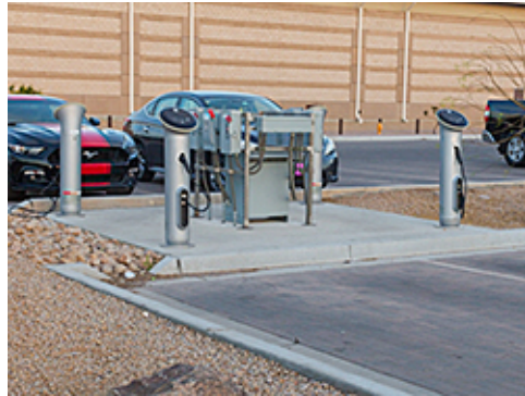
EV Station Integrated with Median
