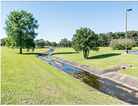
Base-wide Stormwater System
