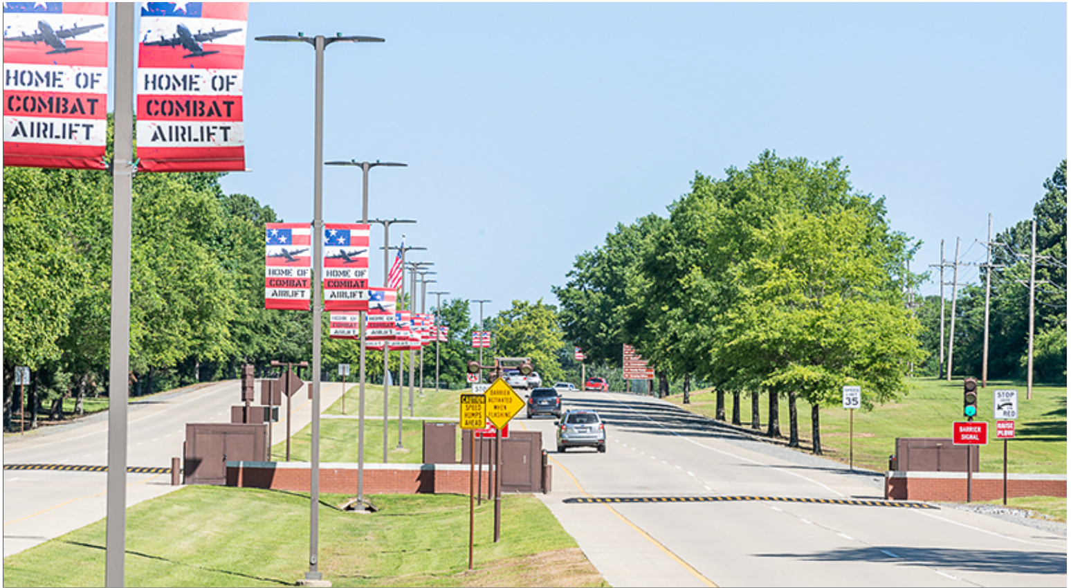
Double Pole Street Lighting
