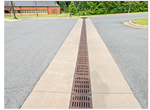
Trench Drain at Parking
