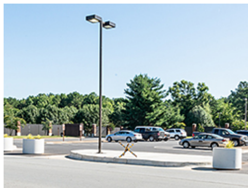
Pole Mounted Fixtures
