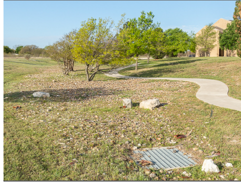
Area Drain and Swale in Landscape
