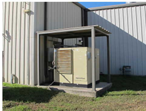
Pad Mounted Equipment
