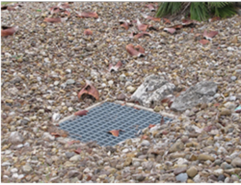
Area Drain Inlet
