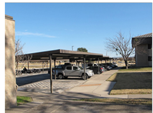
Solar Array and Shading
