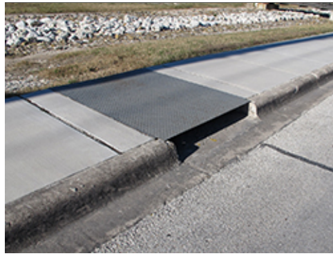
Curb and Gutter Inlet
