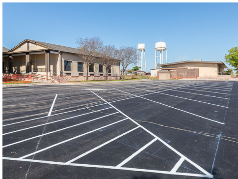
White Striping on Asphaltic Paving
