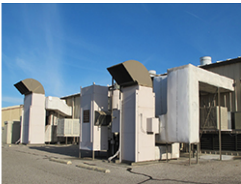
Ground Mounted HVAC equipment
