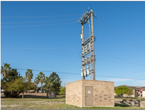
Above-Ground Electrical Service
