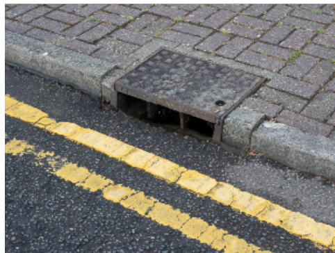
Storm Drain at Street
