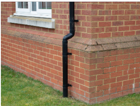
Downspout to Underground Drainage
