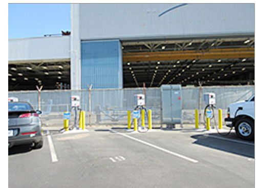
EV Charging Stations
