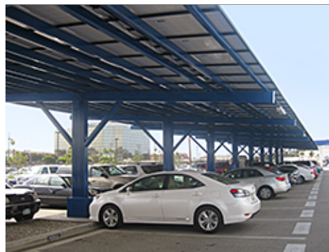
Solar PV Array and Shading
