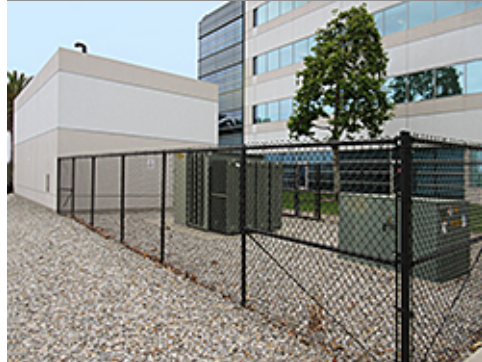
Fenced Utility Yard
