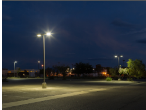
Parking Lot Pole Lighting with LED luminaires
