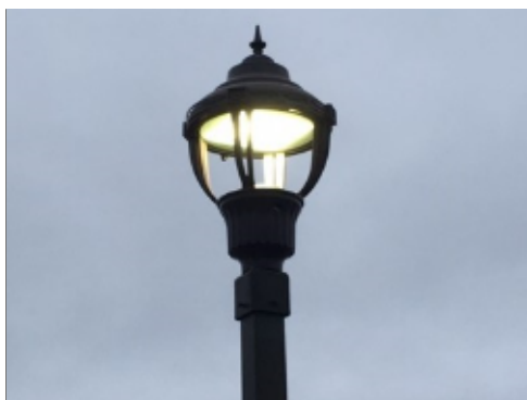
Decorative LED Street Lighting
