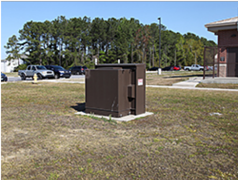
Pad Mounted Cabinet
