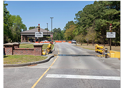
Active Barriers at Gate
