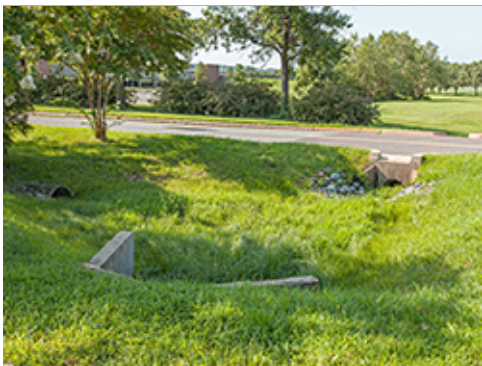
Storm Drainage Elements
