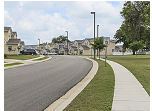
Detached Sidewalk at Group 4
