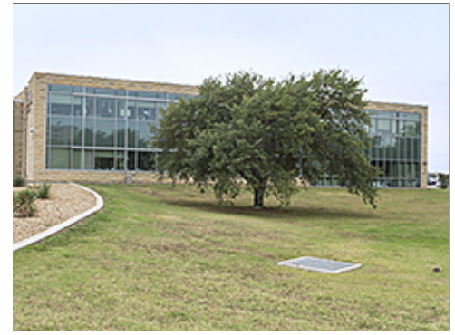
Storm Drainage Inlet
