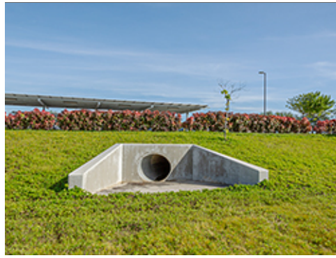
Stormwater Pipe at Group 2
