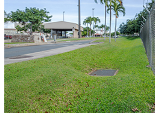
Coordinated Storm Drainage
