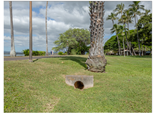
Stormwater Pipe along Walking Trail
