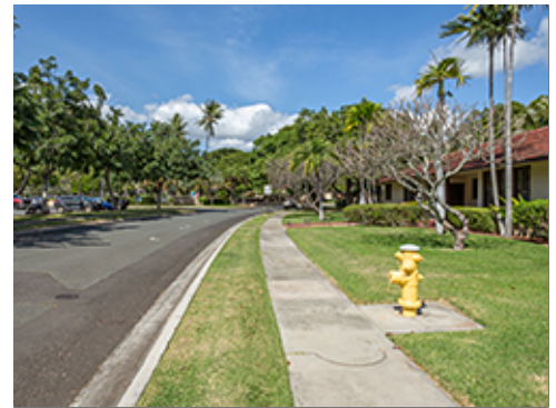
Fire Hydrant Accessible
