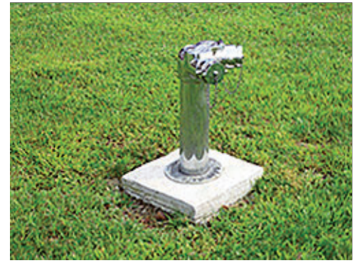
Fire Service Standpipe
