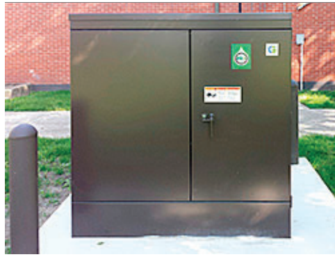
Painted Electric Cabinet
