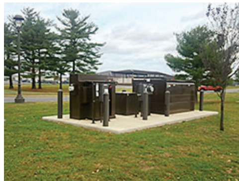
At-Grade Electric Service
