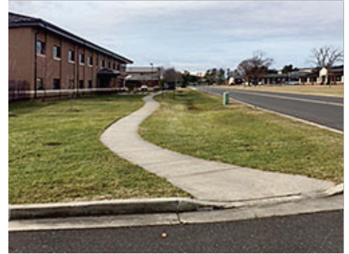
Detached Concrete Sidewalk
