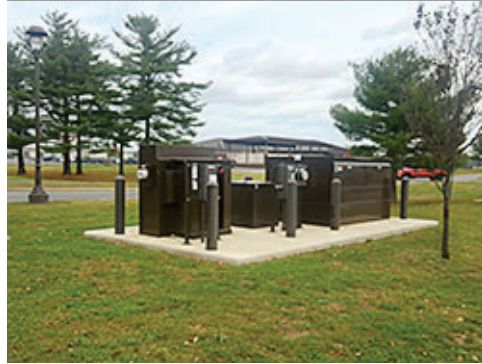
At-Grade Electric Service
