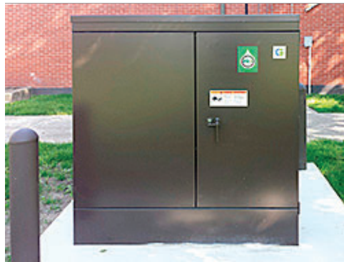
Painted Electric Cabinet
