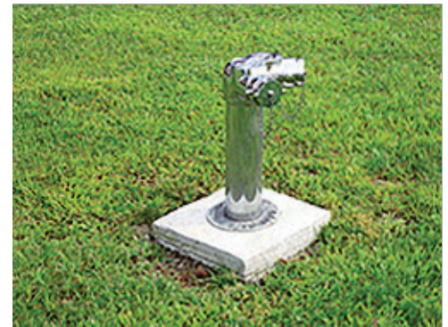
Fire Service Standpipe
