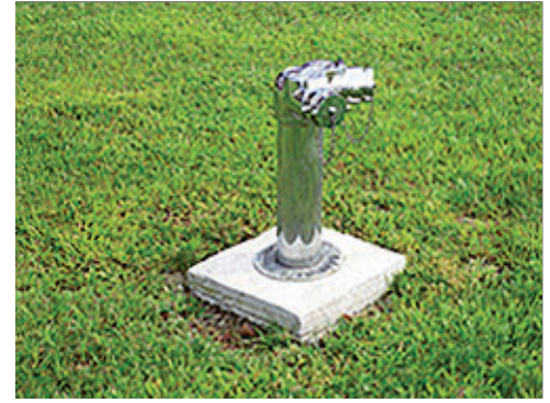
Fire Service Standpipe
