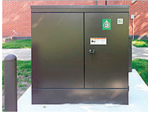
Painted Electric Cabinet
