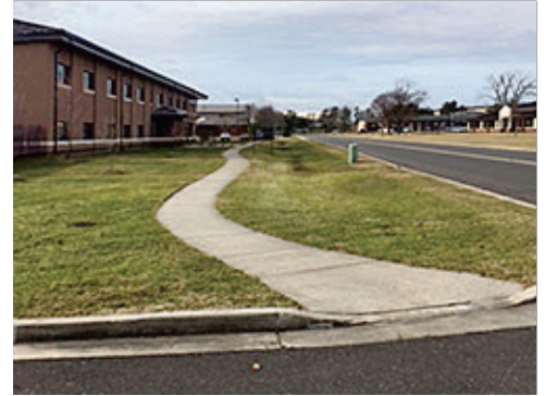
Detached Concrete Sidewalk
