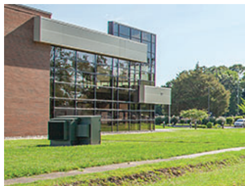
Pad Mounted Transformer
