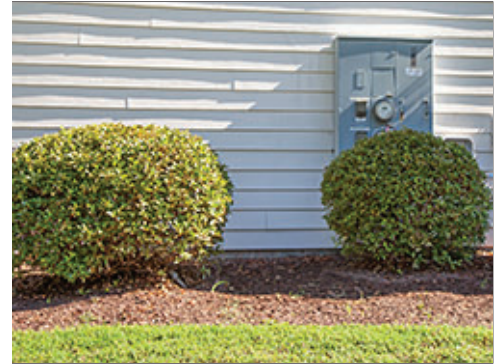
Landscape Screen at Electrical Cabinet
