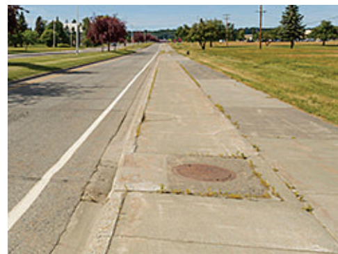
Storm Inlet with Access Cover
