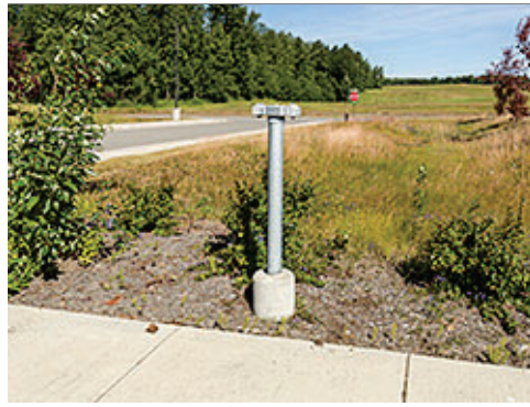
Electric Service for Vehicle Block Heater
