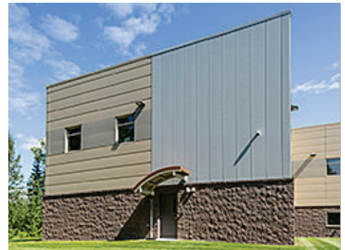
Wall Mounting at Secondary Entrance
