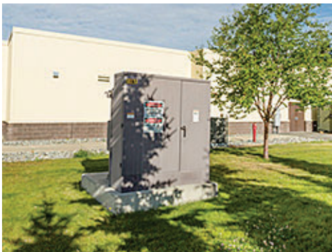
Pad-Mounted Electrical Cabinet
