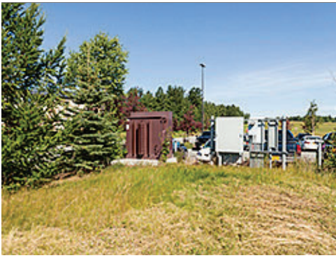
Electrical Gear Behind Screening
