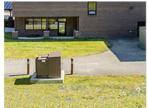
Electrical Gear at Access Drive
