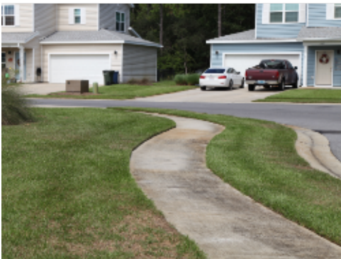
Detached Sidewalk along Roadway
