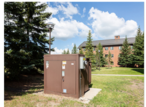
Cabinet Behind Evergreen Screening
