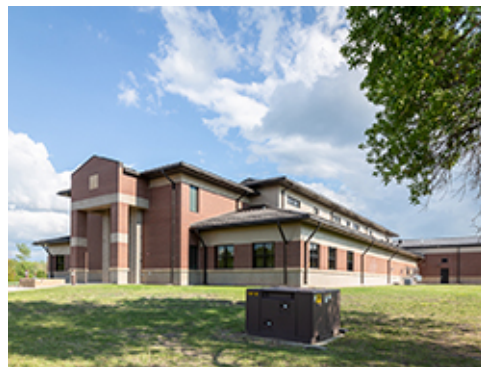
Inconspicuous Utility Cabinet
