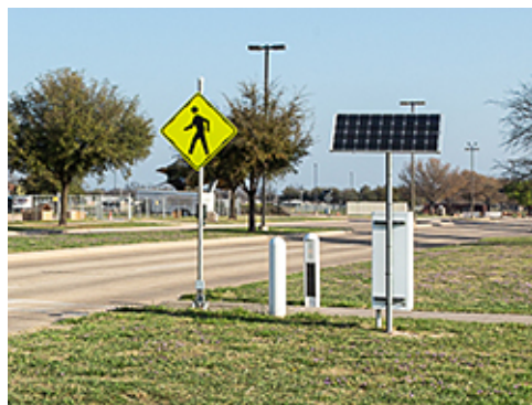
Ground Mounted Equipment
