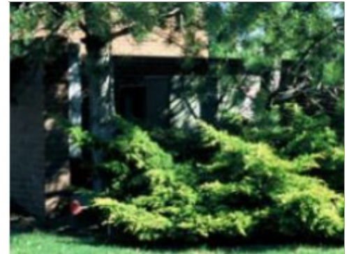
Transformer hidden by landscape screening
