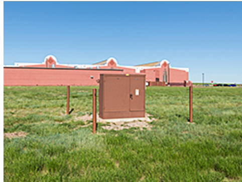
Remotely Located Utility Cabinet
