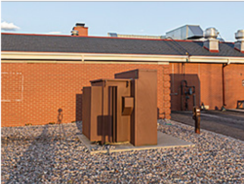
Adjacent Standard Color Utility Cabinet
