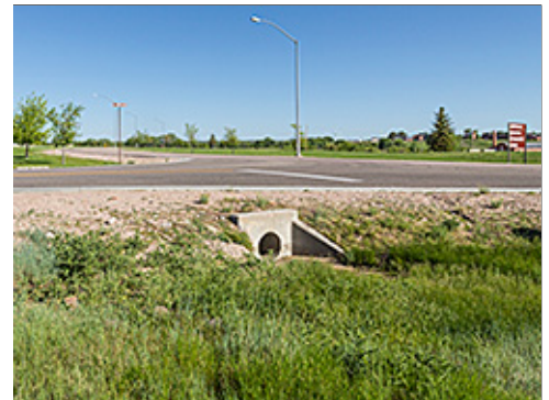
Street Stormwater Feature
