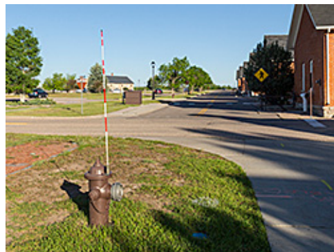
Hydrant with Snow Marker
