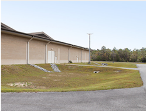
On-Site Engineered Stormwater System
