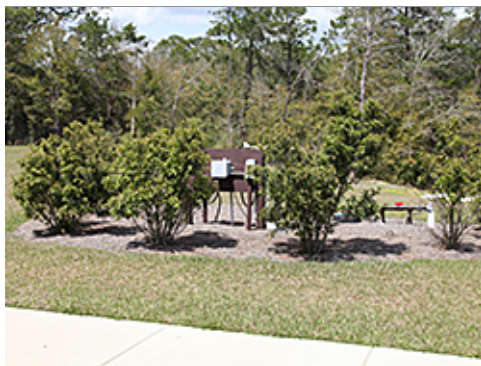
Screening of Equipment
