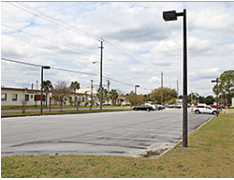
Parking Lot Light Fixture
