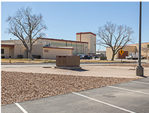
At Grade Equipment Cabinet
