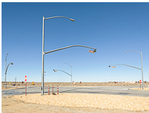
Single Head Fixture at Intersection
