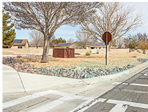
Electric Cabinet in Street Frontage
