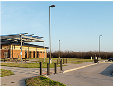
Combined Parking and Pedestrian Lighting
