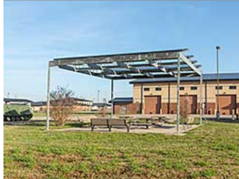
Solar PV Panels on Shade Structure
