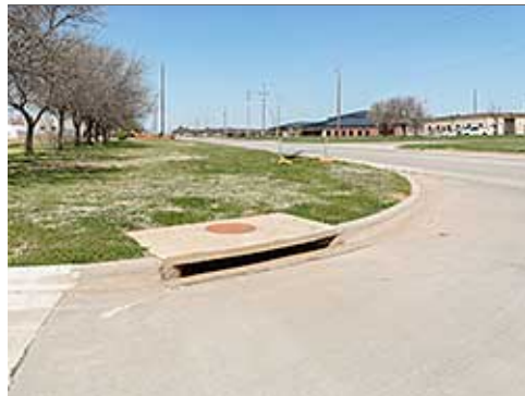
Inlet to Subsurface System
