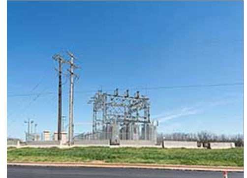
Above Grade Utility Gear and Service Lines
