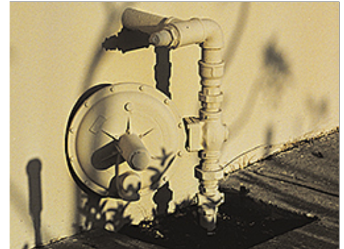
Piping Painted to Match Wall
