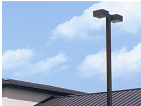
Parking Lot Fixture
