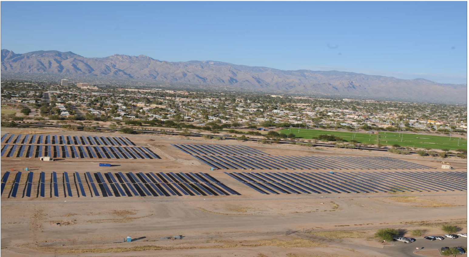
Ground Mounted Solar Array
