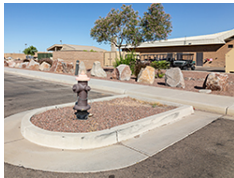
Fire Service Element
