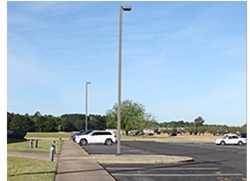
Shoebox Fixture in Parking Area
