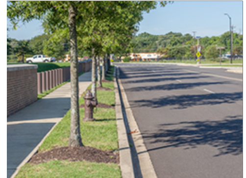
Fire Hydrant with Standard Color
