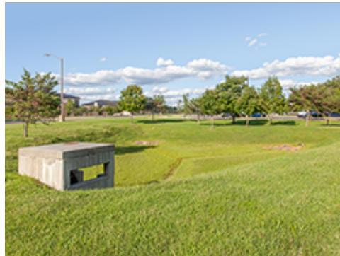
Detention Basin with Overflow Element
