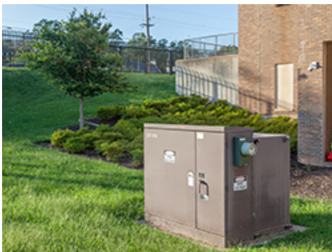
Electrical Service Cabinet with Meter
