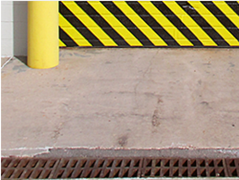
Trench Drain Connected to Storm Drainage
