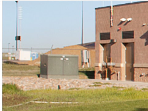
Pad Mounted Cabinet at Group 3
