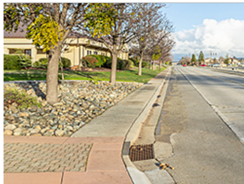
Integrated Storm Inlet
