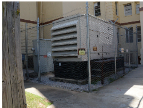
Fencing at Equipment
