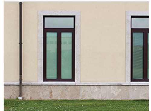
Roof Drainage Directed Underground
