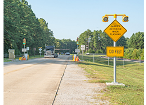
Traffic Control Device
