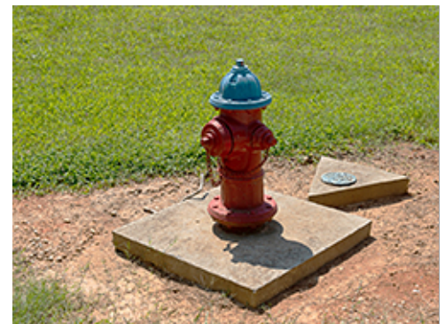
Fire Hydrant Service Line
