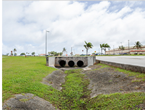
Stormwater Pipe at Street
