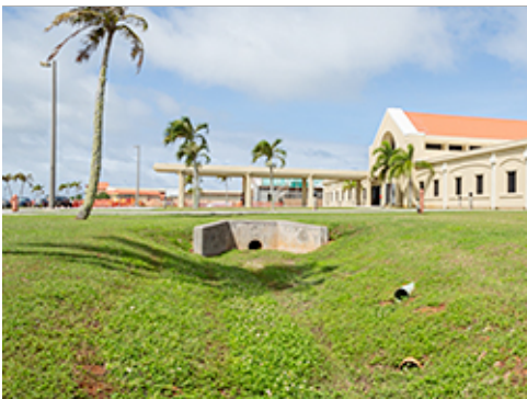
Stormwater Providing Irrigation
