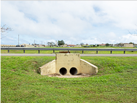
Stormwater Pipe at Street
