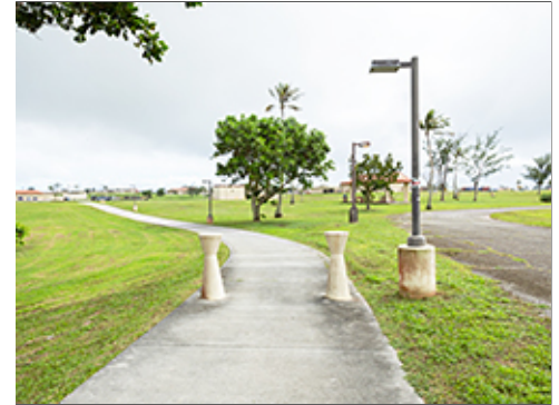
Pedestrian Height Light Fixtures
