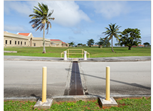
Inlet and Grate
