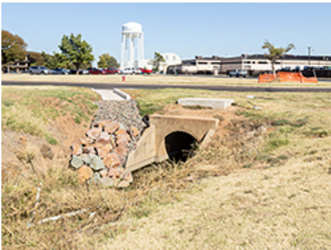
Stormwater Pipe at Street
