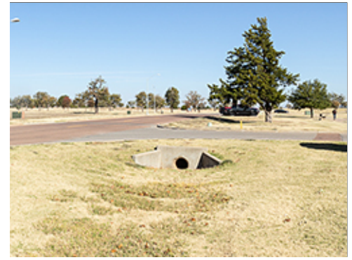
Stormwater Pipe at Street
