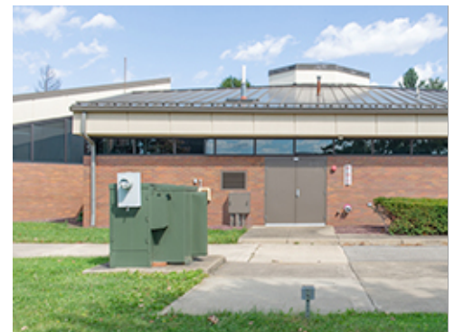
Buried Utility Lines to Cabinet at Group 1
