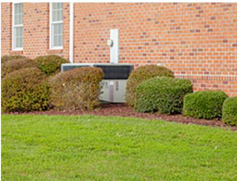
Screening Mechanical Equipment
