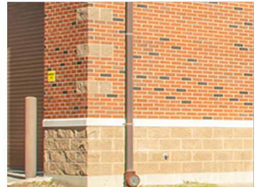
Group 2 Base in CMU and Matching Quoins
