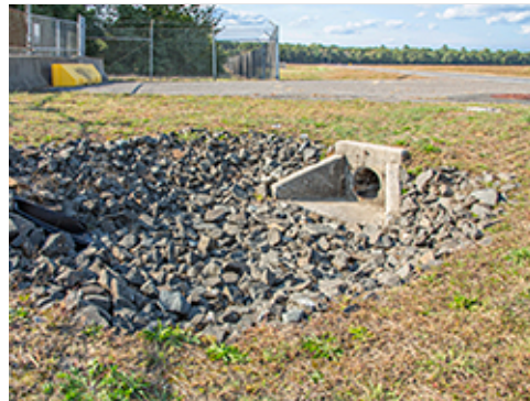
Rip-Rap Coarse Rubble at Outlet
