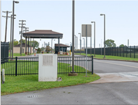
Underground Electric Service at Group 1
