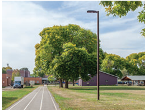
Lighting at Running Track
